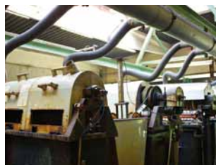
Continuous galvanizing line
